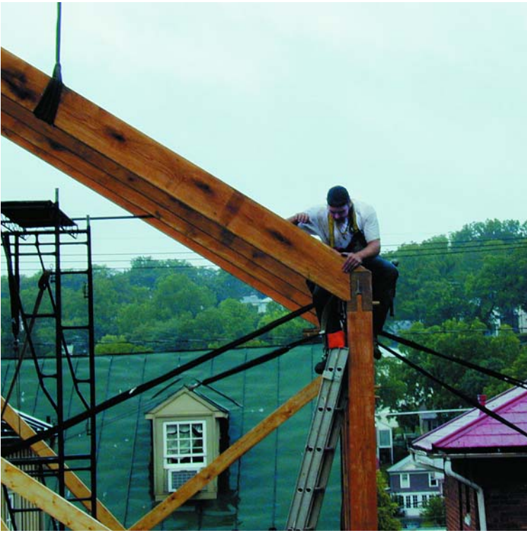
Fig. 3. Fitting the white oak rafters. Support is at ledge in plate and combines with support at underslung ridge to eliminate rafter thrust.
